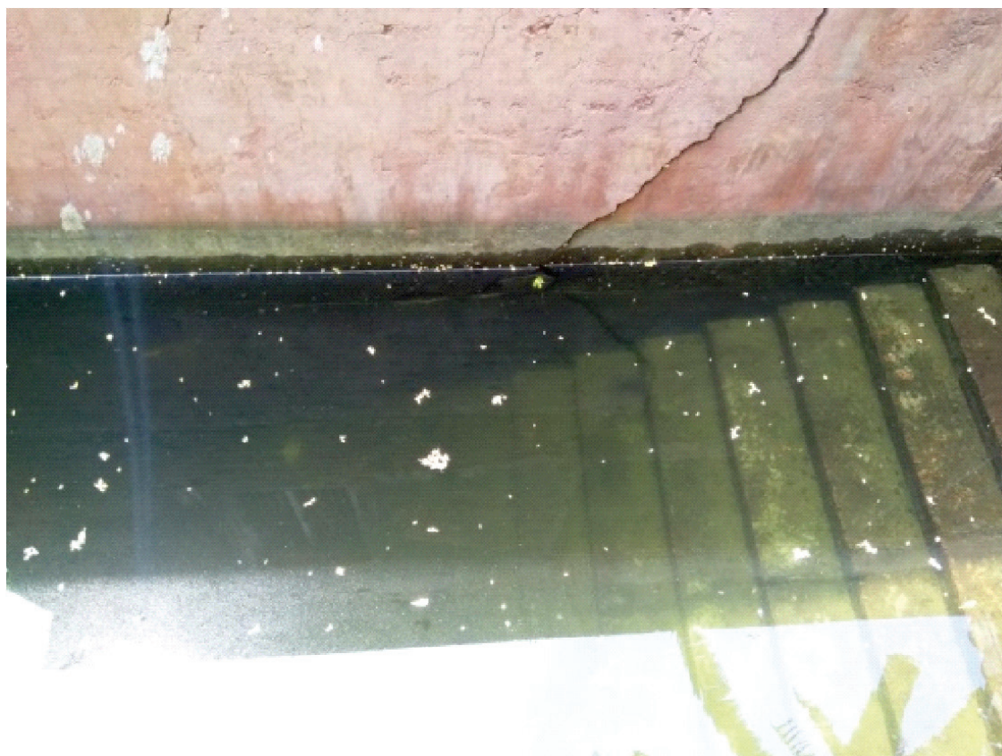
Figure 16: Stairs under water (2008)
